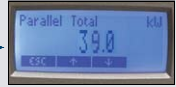
Display full system output from any UPS
